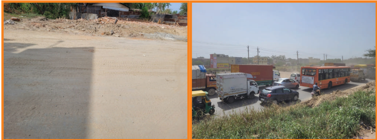
Figure 7: High Silt Load, Poor Road condition and improper disposal of muck from excavation (NIA to Karnal road)
